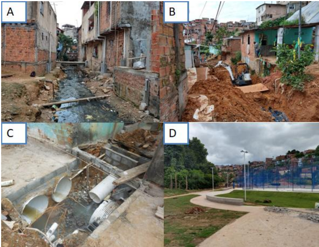
Figure 2: A & B) An open sewer between households in the study area, C & D) The study area undergoing environmental modification i.e. channelling of the drainage into a major junction, and the construction of community square, roadway and sidewalk.
