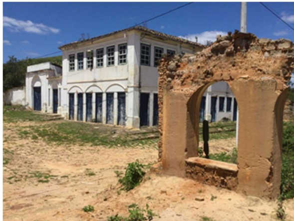
Fig. 9 A few old commercial buildings are still intact whereas others are in thorough ruin
