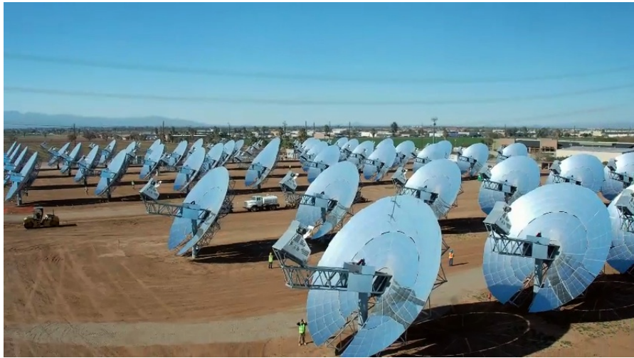
Figura 15 – Maricopa Solar Project
