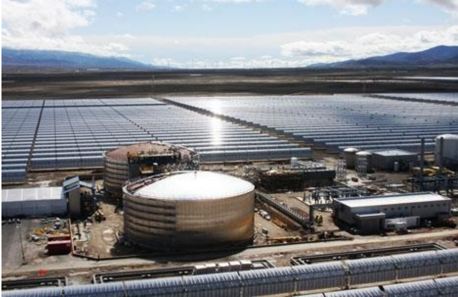
Fig. 17. Molten salt thermal storage, Source: SOLAR MILLENNIUM, 2008
